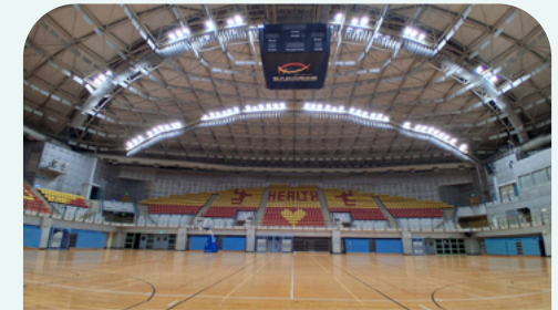
LED lighting upgrade at the 3F Main Stadium of the NTU Sports Center.
